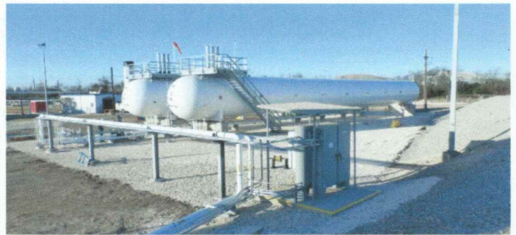
XL Industrial Services mechanical, electrical, and coating employees provided full-service installation of a two-tank butane blending system.
